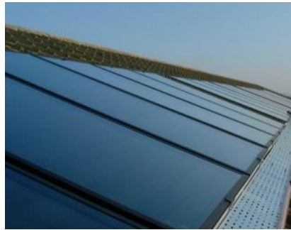
Solar thermal hot water
