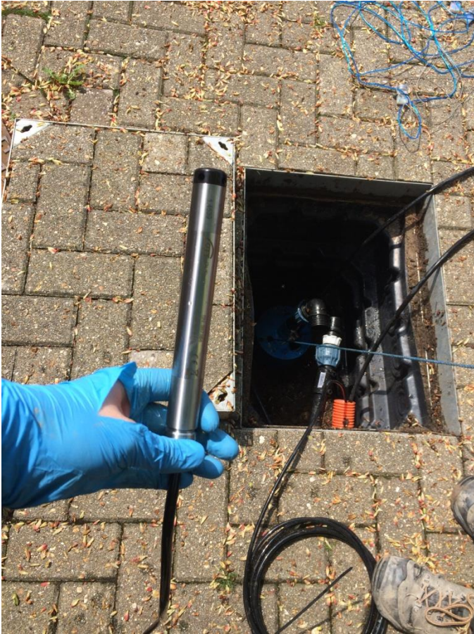
Abstraction Borehole (BH1). No iron build-up after 6 months.
