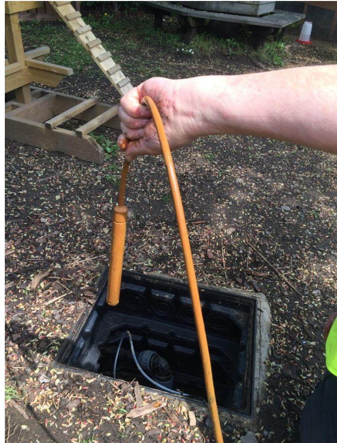
Injection (return) borehole (BH2). Iron precipitation on the logger device.
