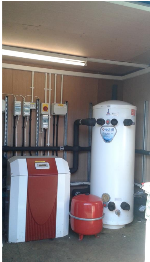
Heat pump and buffer tank
