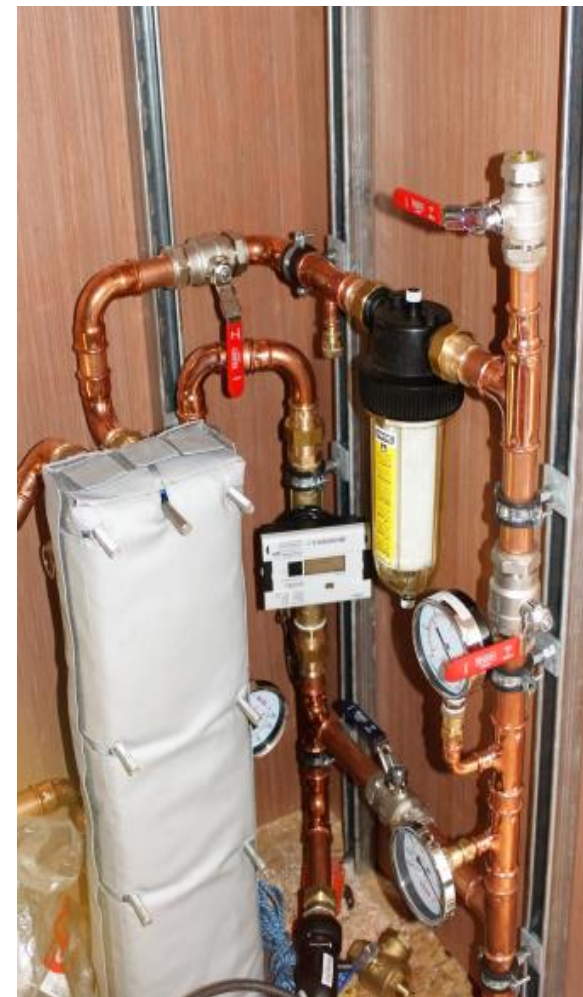
Heat exchanger, filter and flow meter
