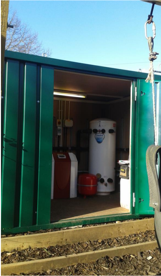
Housing with heat pump system
