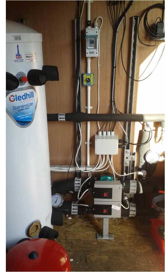
Delivery pumps with loggers/metering
