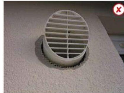
Figure 34: Unsealed extract fan in a bungalow
