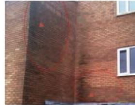
Figure 5: mould on saturated brickwork
