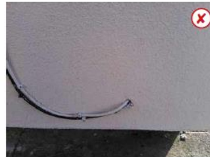
Figure 36: Unsealed wire penetration
