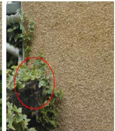
Figure 49: Close proximity of plant requiring pruning
