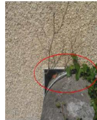
Figure 48: Plant growth allowed by poor detailing
