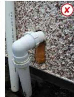
Figure 35: Unsealed pipe penetration
