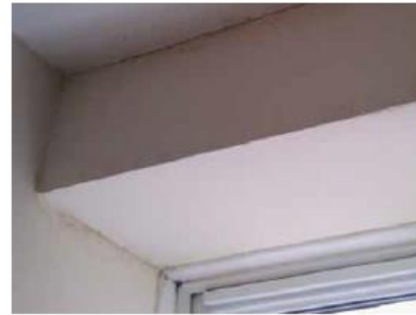
Figure 50: Damp in the kitchen
