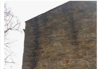
Figure 14: Staining from roof water run off
