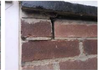
Figure 12: Cracked and missing
