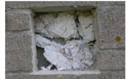
Figure 4: Example of saturated insulation
