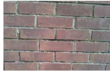
Figure 11: Erosion of mortar by weather
