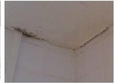
Figure 51: Damp in the bathroom
