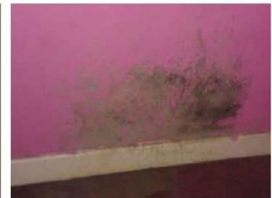
Figure 53: Damp behind a bed, removed for inspection
