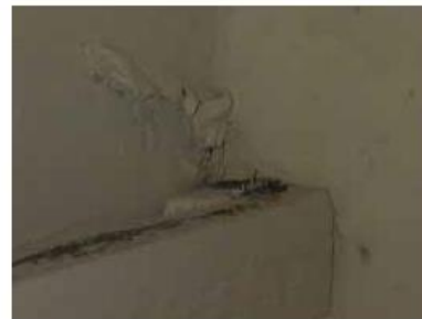
Figure 52: Damp in the wardrobe
