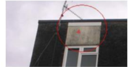
Figure 6: mould on saturated render panels
