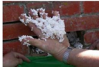
Figure 3: Example of saturated insulation
