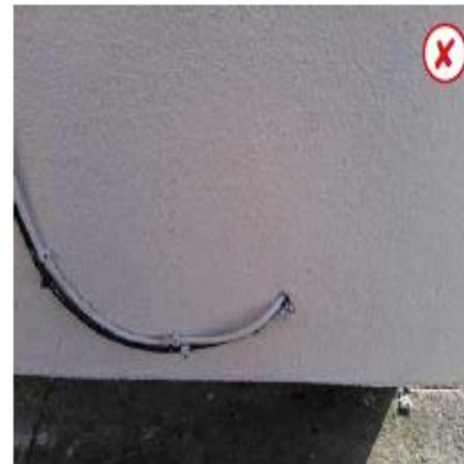
Figure 36: Unsealed wire penetration
