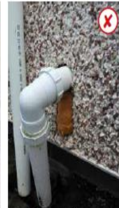
Figure 35: Unsealed pipe penetration
