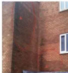
Figure 5: mould on saturated brickwork
