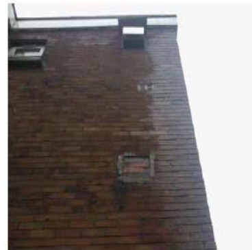
Figure 13: Wall staining from water blown off the roof
