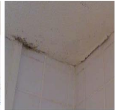
Figure 51: Damp in the bathroom
