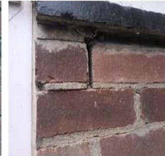
Figure 12: Cracked and missing
