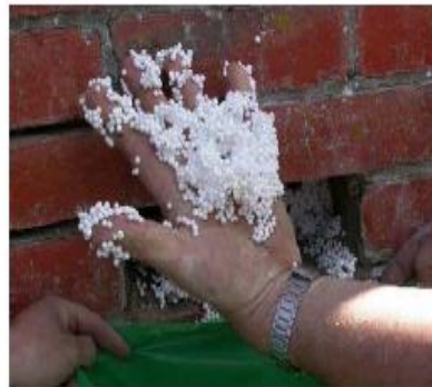
Figure 3: Example of saturated insulation
