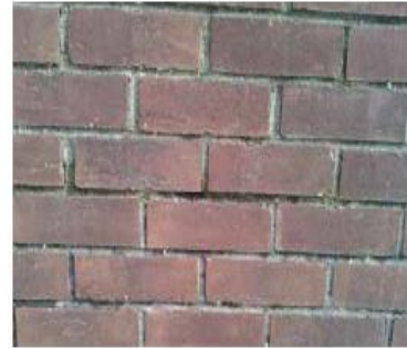
Figure 11: Erosion of mortar by weather
