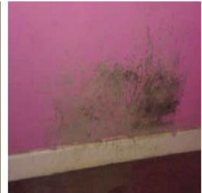
Figure 53: Damp behind a bed, removed for inspection
