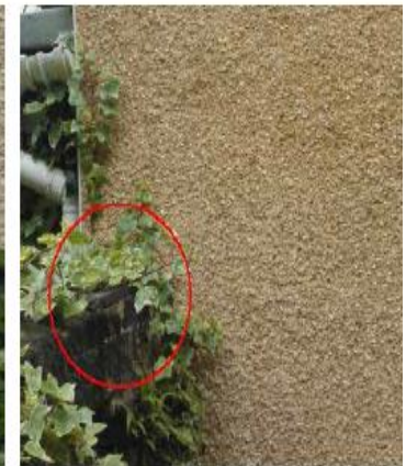
Figure 49: Close proximity of plant requiring pruning
