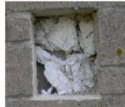
Figure 4: Example of saturated insulation
