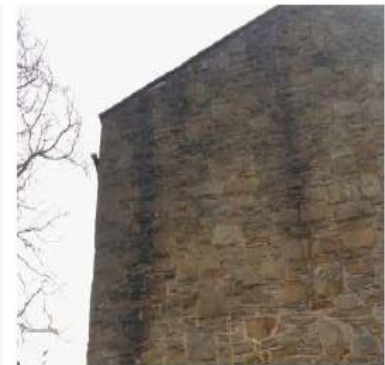
Figure 14: Staining from roof water run off
