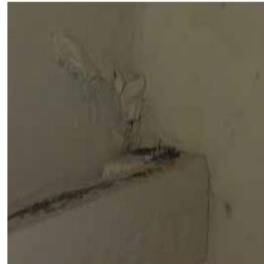
Figure 52: Damp in the wardrobe
