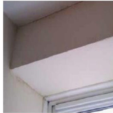
Figure 50: Damp in the kitchen
