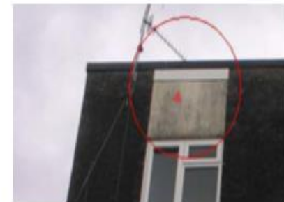
Figure 6: mould on saturated render panels
