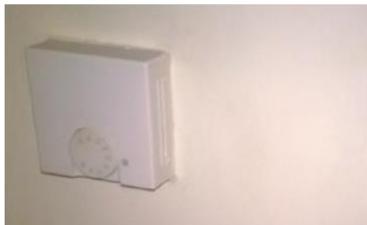
Flat Hall (main) Thermostat
