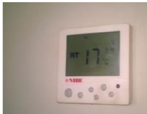
House Hall (main) Thermostat
